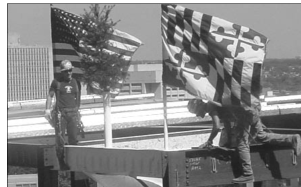
Construction workers lay the final beams at the topping out ceremony for the new Dental School facility.
