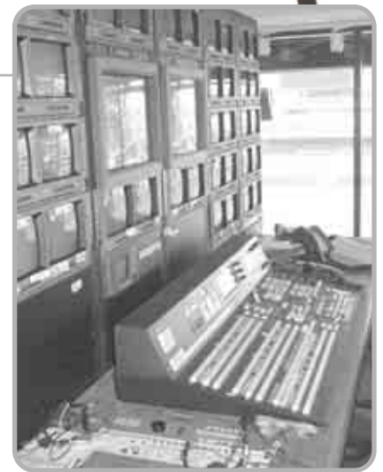
control room design
