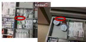
Omnicell issues: broken bins and missing labels are not fixed due to RN's lack of free time (4T)
